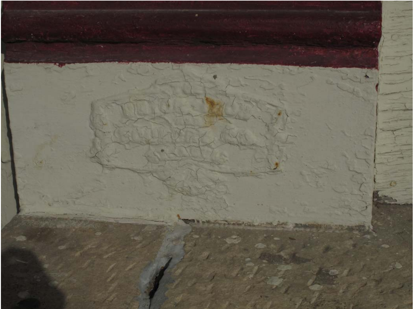
Photograph 92-00518-007 - Detail of stamp on left column on 202 storefront, looking east (McCarley, September 20, 2011)
