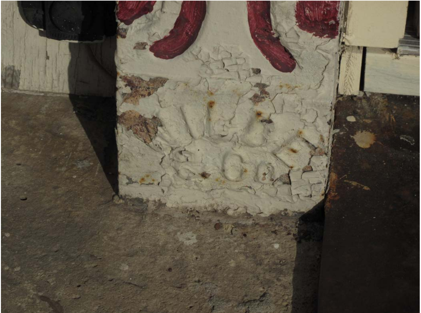
Photograph 92-00518-009 - Detail of stamp (Wilde & Co) on middle column on 202 storefront, looking east (McCarley, September 20, 2011)
