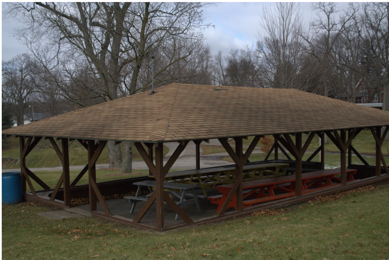
Photograph 92-00805-002 - Shelter 1 (S1) in Section 1 (former wading pool converted to picnic shelter), looking northwest (December 2014)
