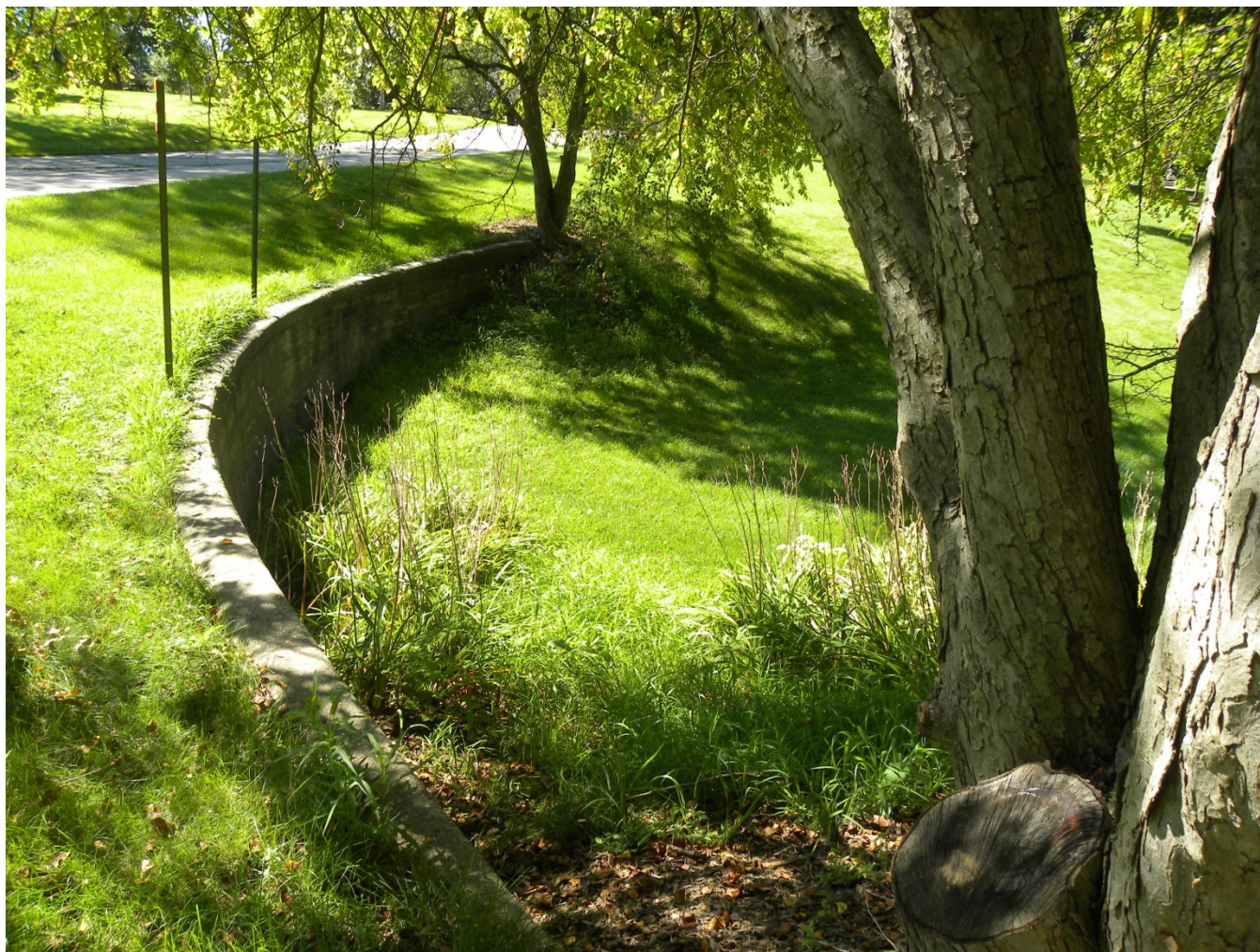
Photograph 92-00805-004 - Concrete retaining wall (1928 date on top) along west edge of Jefferson/Washington loop, looking south (July 2015)
